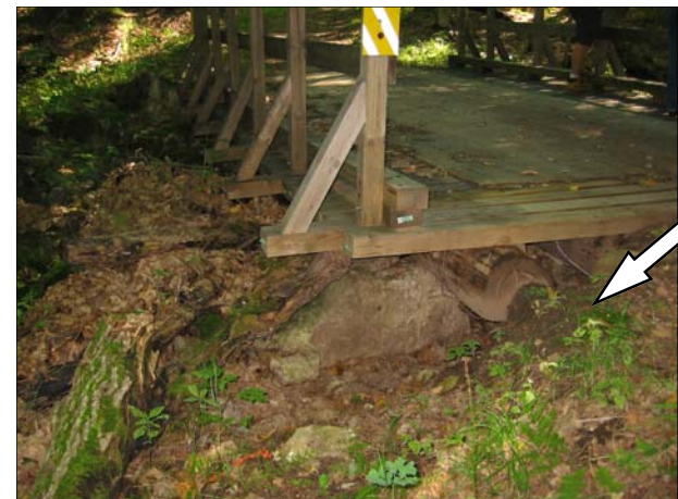
Eroded approach to the bridge.
